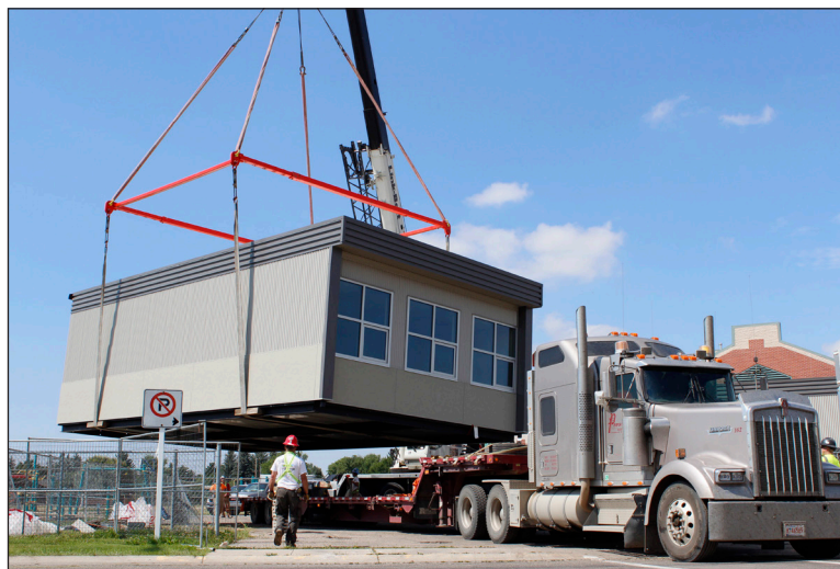
One of two modular classrooms is moved into place at Jennie Emery Elementary School in Coaldale in August 2014.
